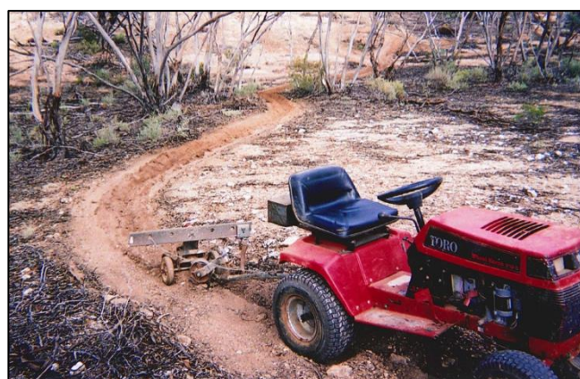
Figure 9: Small grader towed by mini-tractor with little ripper attachment in use, cutting a water runoff drain.
